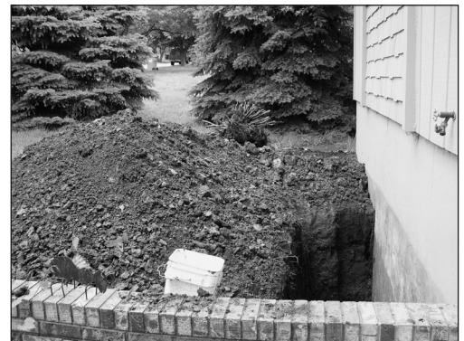
Photo 1. Excavation of the basement wall shows no retarder and causes much disruption of landscape for repair.
