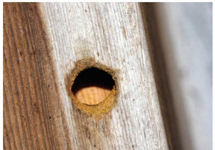
Figure 4: Carpenter bee tunnel entrance
