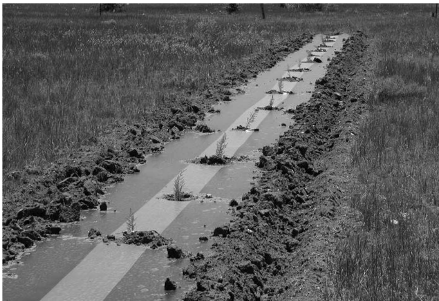
Figure 4. Properly installed fabric pulled tight to avoid wind, with dirt placed on edges and holes for seedlings large enough to avoid girdling.
