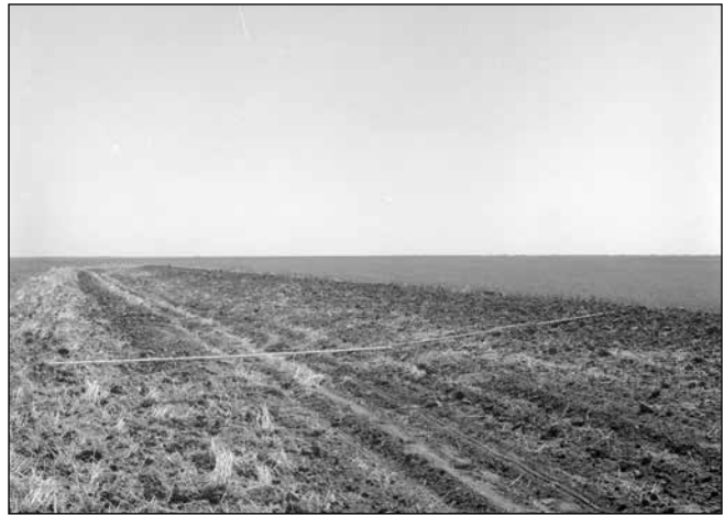
Photo 4. The cross-section shape of a terrace more than 10 years old depends on practices used to maintain the terrace. After maintenance, this terrace has a good shape with adequate width and height, and a smooth channel and ridge.
