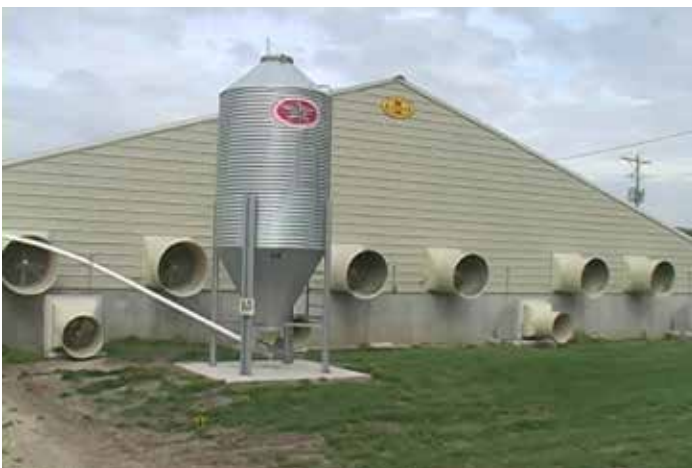
Figure 3.10. Swine barn exhaust fans. Vents that provide clean makeup air are located on the opposite side of the building.
