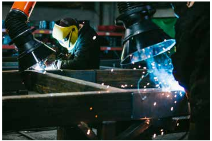
Figure 8.4. Local exhaust hoods remove welding fumes and help keep the workplace air clean.
