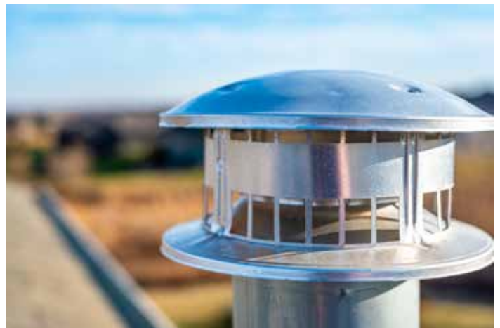
Figure 13.4. Fuel-fired appliances should be vented outdoors.
