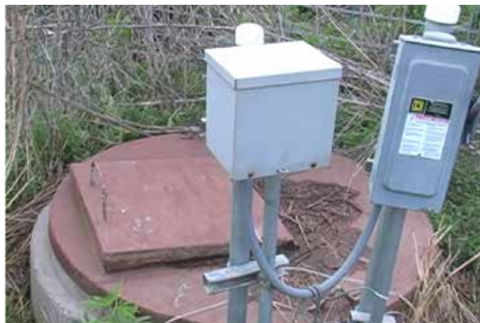
Figure 4.2. Low oxygen levels and hazardous gases are common in water wells and cisterns.
