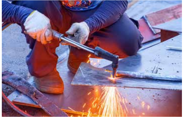
Figure 1.7. Workers are exposed to fumes and gases during hot work such as torch cutting and welding.
