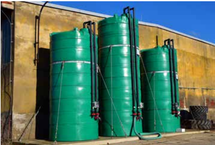
Figure 4.4. Farm storage tanks often contain low oxygen and hazardous gases.
