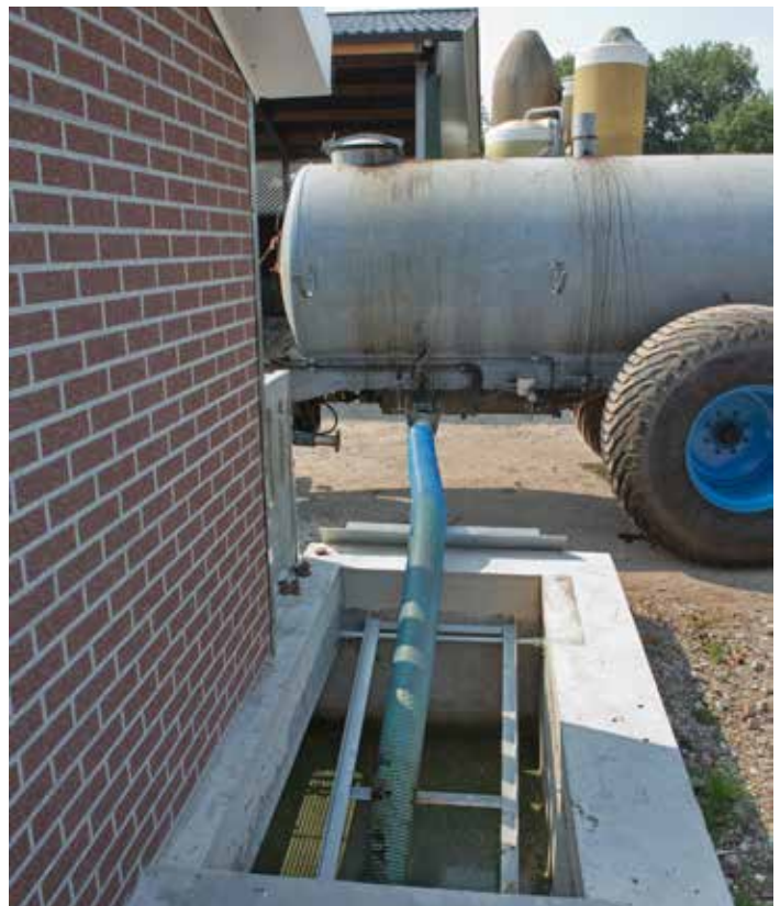
Figure 3.9. Underground manure pit being pumped. Toxic gas concentrations can increase in occupied areas of barns when waste is flushed, agitated, or pumped.
