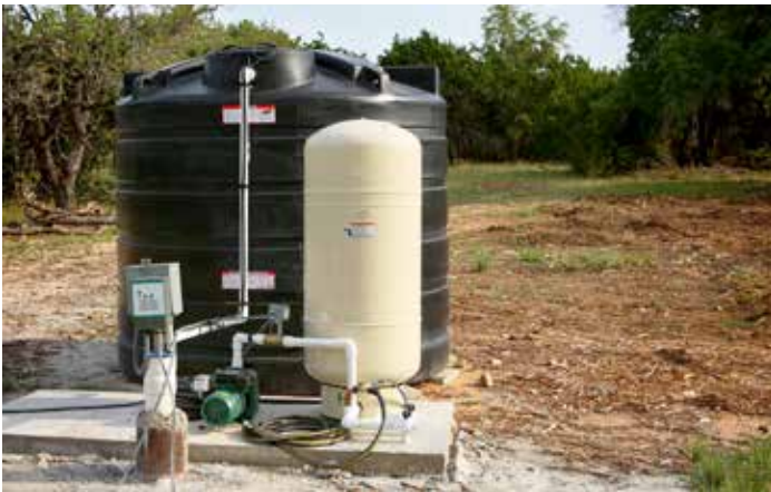
Figure 11.1. A confined space is large enough to enter fully and work inside. The black storage tank of this water well is large enough to enter. Thus, it may be considered a confined space if it also has limited entry/exit and is not designed for continuous occupancy. In contrast, the light-colored pressure tank is not a confined space because it is too small to enter and work inside.
