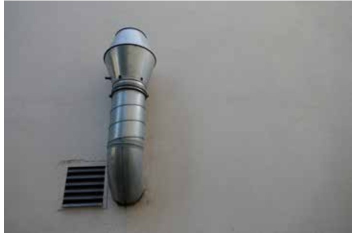
Figure 7.11. Tailpipe-exhaust extraction systems must be vented outdoors, away from building air intakes.
