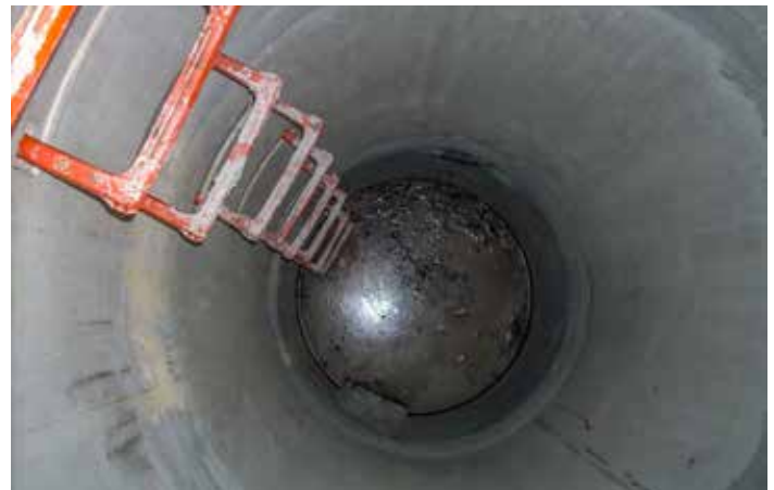
Figure 11.7. A confined space may be permit-required if it has the potential for a hazardous atmosphere. Underground confined spaces often contain low oxygen concentrations or asphyxiating gases.
