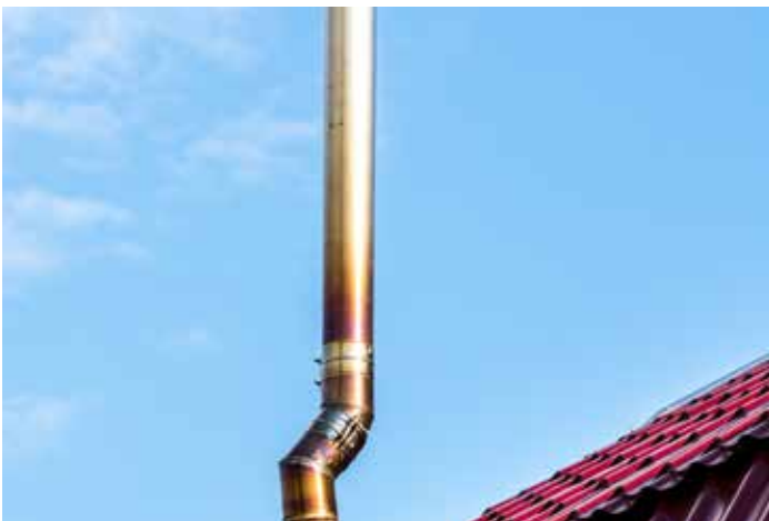
Figure 7.7. Flues from fuel-burning appliances should exhaust combustion gases away from outdoor air intakes.
