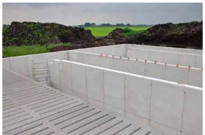
Figure 3.4. This barn floor is under construction. Note the deep manure storage pits directly beneath the slatted floors.
