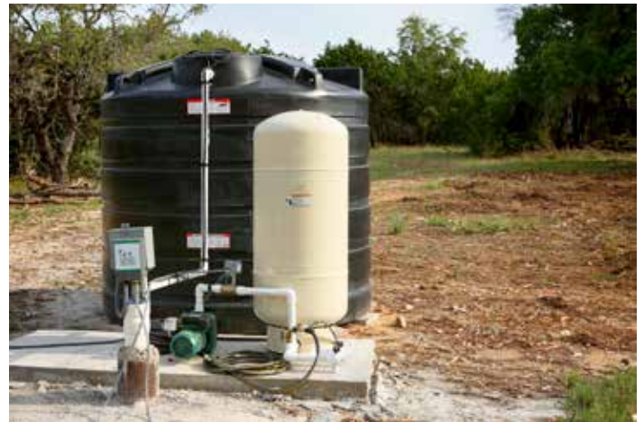
Figure 4.5. Even water tanks (shown here in black) may contain oxygen-deficient air.
