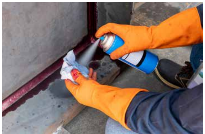
Figure 1.9. Some solvents and maintenance chemicals require extra ventilation and protective equipment.
