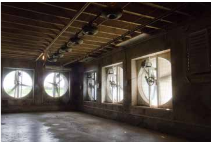
Figure 13.2. Well-designed ventilation systems reduce airborne contaminants in livestock barns. (Credit: USDA)
