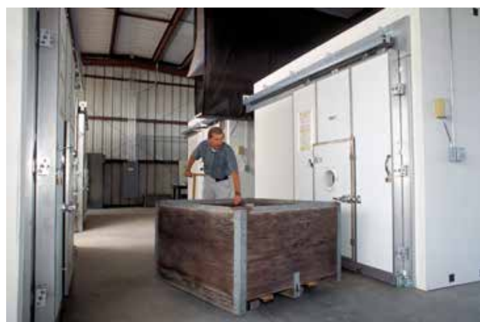
Figure 4.15. Controlled atmosphere storage rooms (the large white chambers in the image) reduce oxygen levels to preserve agricultural products. (Credit: Agricultural Research Service)
