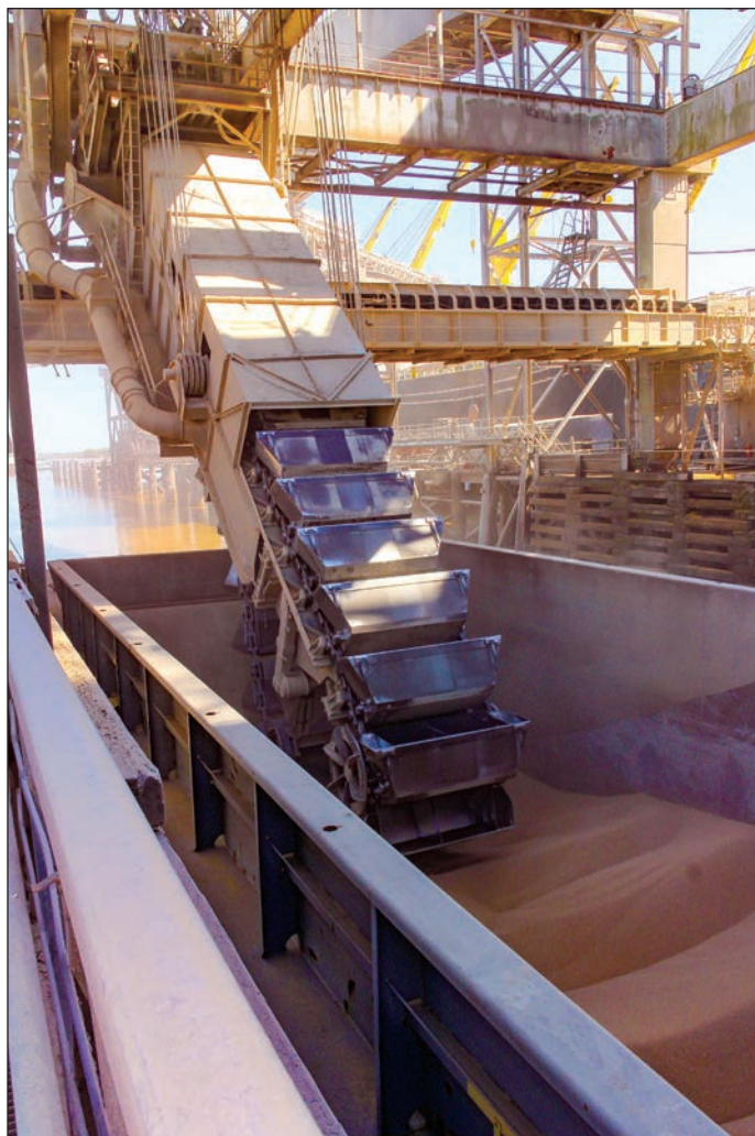
Figure 1. Grain is unloaded from a barge on the Mississippi River using a “marine leg” bucket elevator at the Cargill grain export terminal in Westwego, Louisiana.
