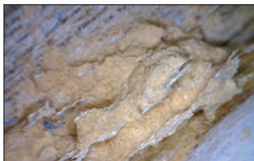
Anobiid powderpost beetle and damage
