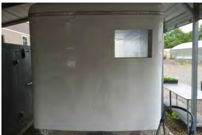
Figure 9. Cut a hole in the front of the trailer for the AC unit with a counter rotating circular saw.
