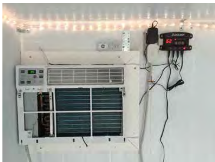
Figure 10. Installation of the AC unit, CoolBot adapter, and lighting.
