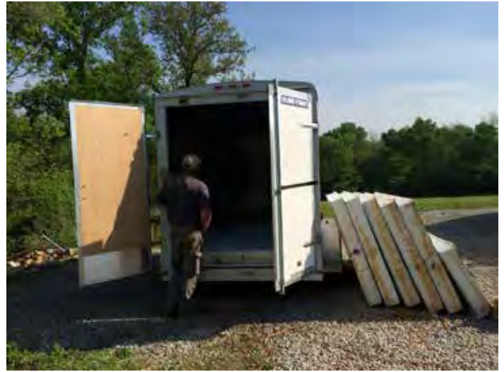
Figure 1. After the floor is finished, the cooler is assembled using the structurally insulated panels (right).
