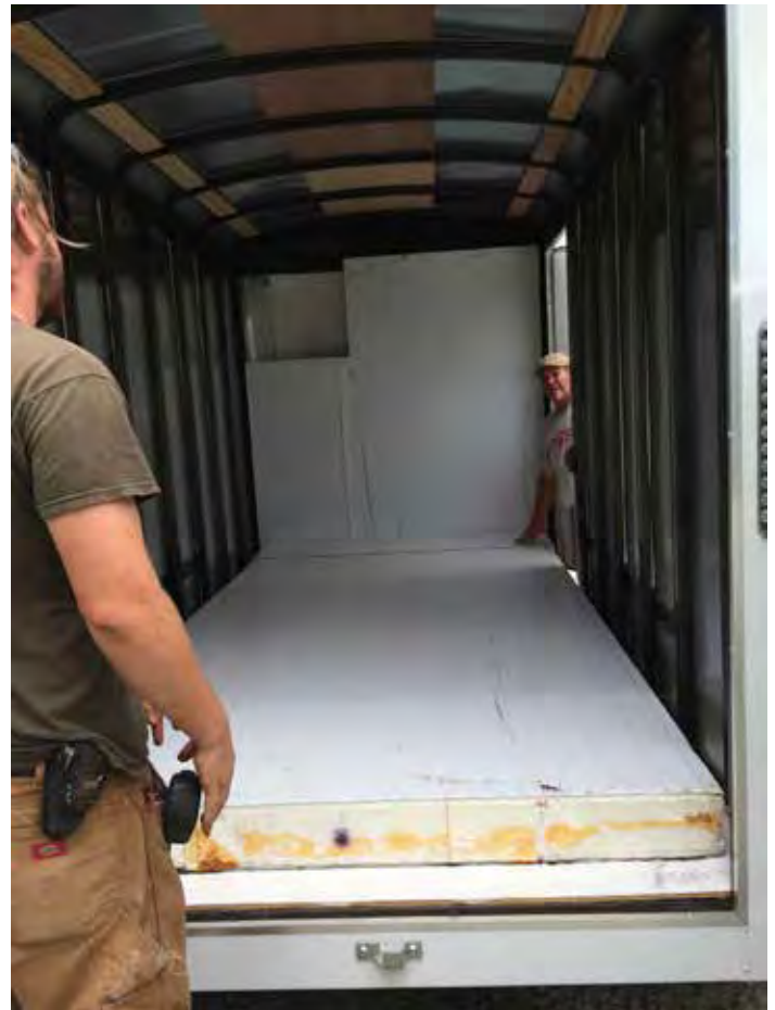
Figure 4. Set the front wall and floor first. The opening at the front should be wide enough to fit the air conditioner unit, 6 inches of insulation, and any airspace outside the insulation.
